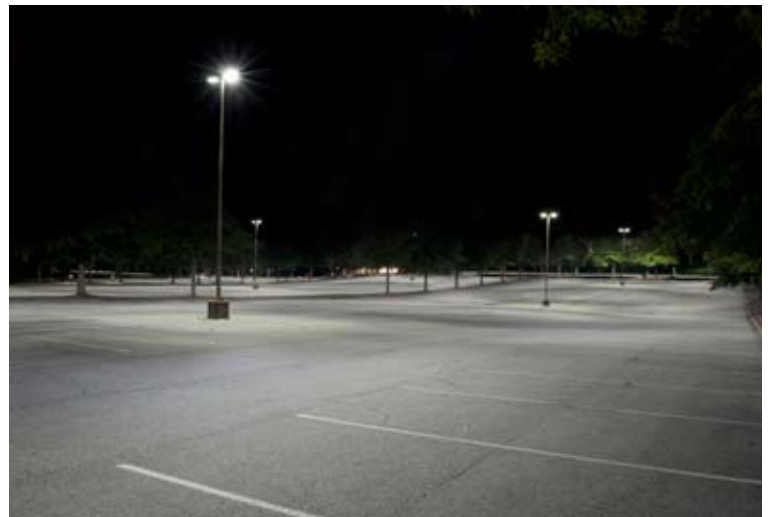
Cimarron 90LED units, double configuration, mounted at 28 ft.
